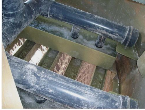
Figure 2. Photograph taken during the full-scale test of the liquid distribution system for a vessel on the OCSD 180,000 CFM odor control system. The test was done to ensure full coverage of the vessel bed below by liquid streams.
