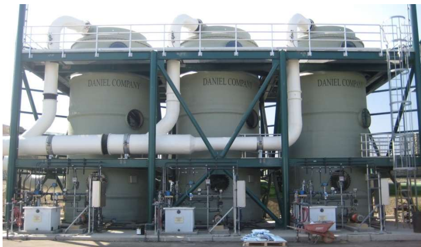
Picture #3: North Central Outfall Sewer Air Treatment Facility - Los Angeles California
