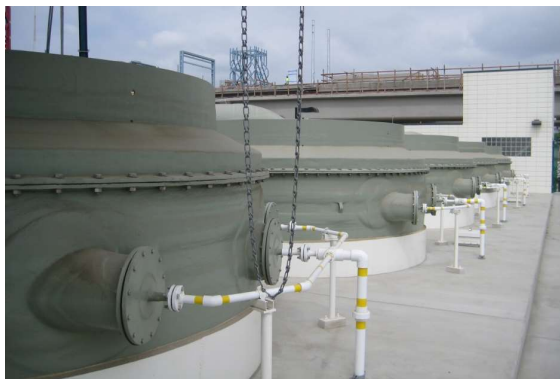
Picture #2: La Cienega and Jefferson Air Treatment Facility - Los Angeles California
