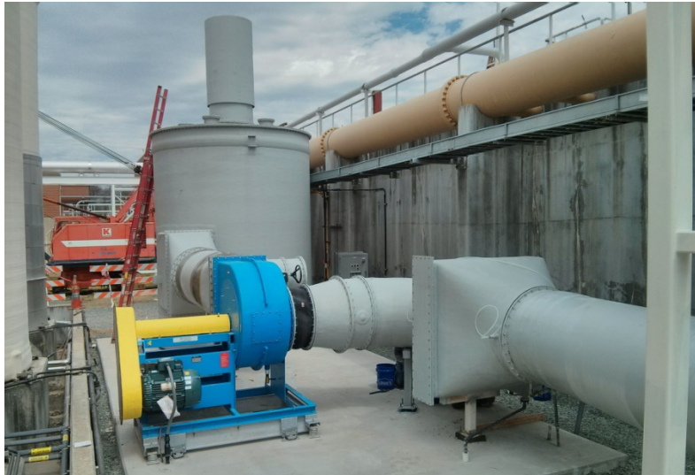
Picture #12: Orange Water and Sewer Authority - Mason Farm WWTP Aeration and Odor Control Improvements. Chapel Hill, North Carolina
