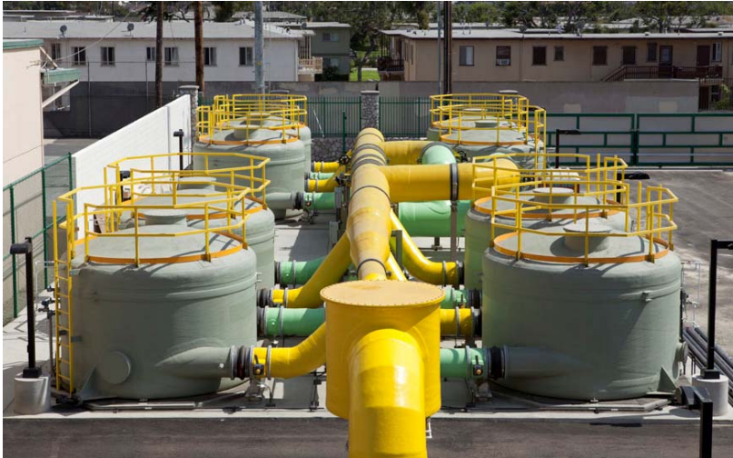
Picture #6: Jefferson/La Cienega - Air Treatment Facility. Los Angeles, California
