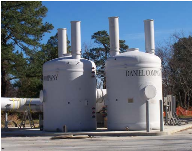
Picture #2: Hampton Roads Sanitation District Nansmond Plant, Virginia
