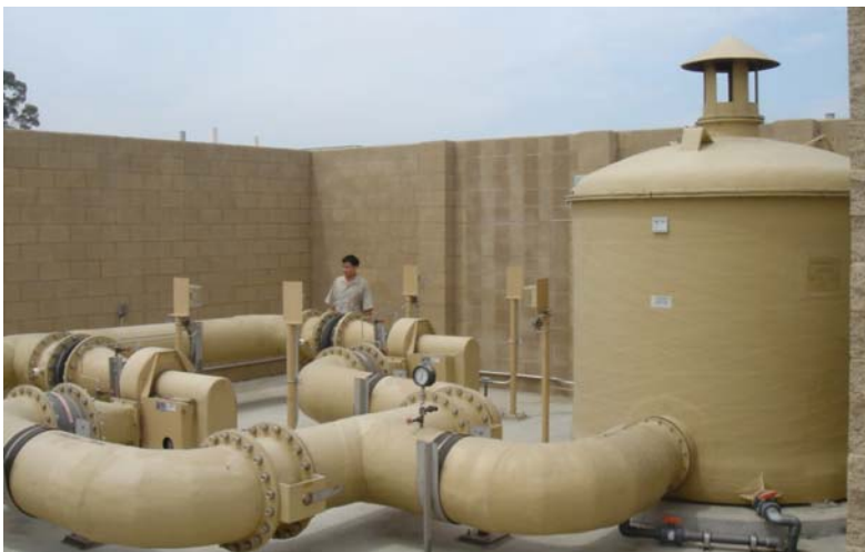
Picture #3: Secondary Treatment Facilities - Stage 3. Carson, California
