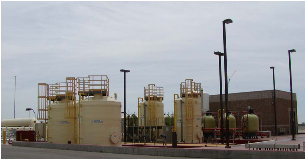
Photo #2: City of Phoenix 91st Avenue WWTP Headworks. Tolleson, AZ
