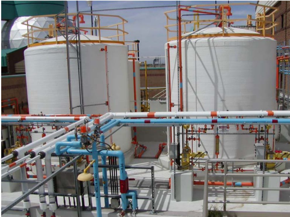
Photo #3: City of Mesa Northwest WWTF, AZ
